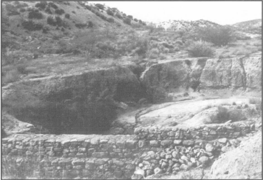
Check Dam in Tonto Basin near Tonto Creek Civilian Conservation Corps Camp. Photo by George D. Hardaway in 1936. Courtesy of the Tonto National Forest.
